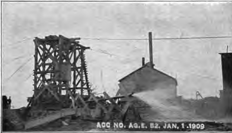
PLATE 82.—Contract 12. Recovering Flooded Shaft by Aid of Air-lift. Trans. Am. Soc. C. E., LXXIII, 1911.
